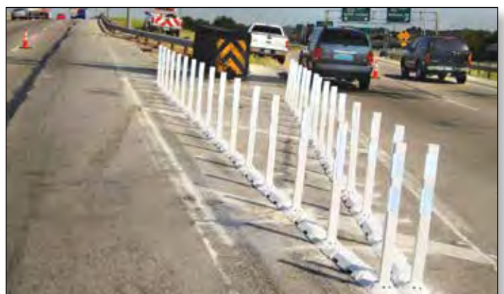
Impact attenuator protection
